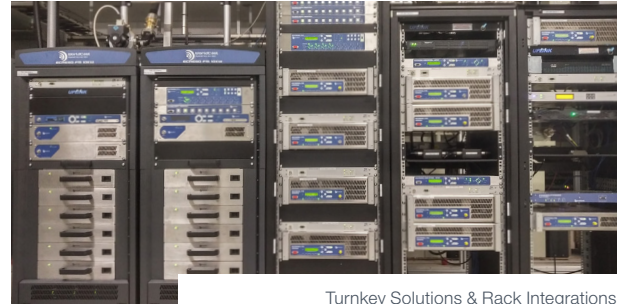
Turnkey Solutions & Rack Integrations
